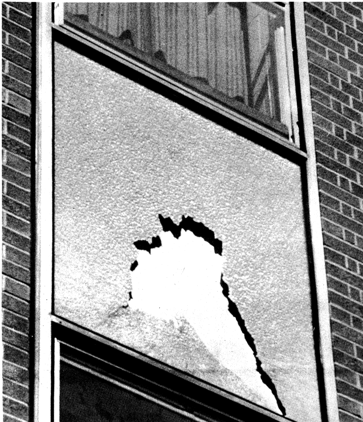
Who should pay for this damage?
