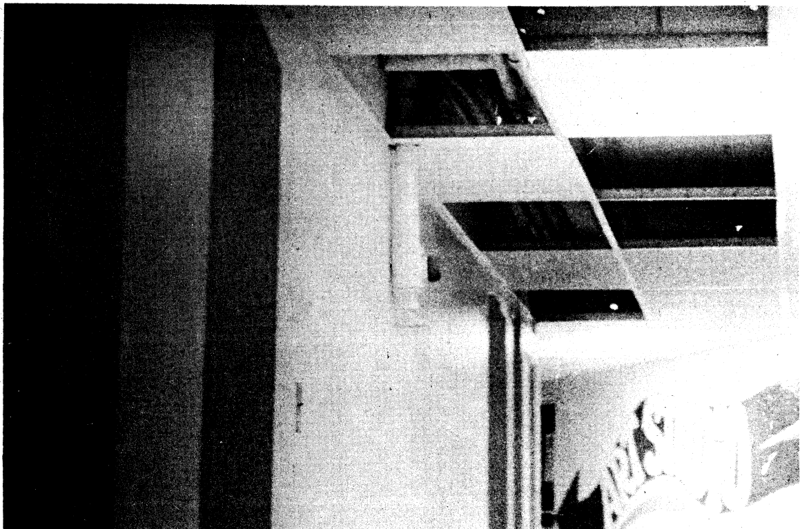
Several ceiling tiles were broken in Glendon Hall last Thursday.
